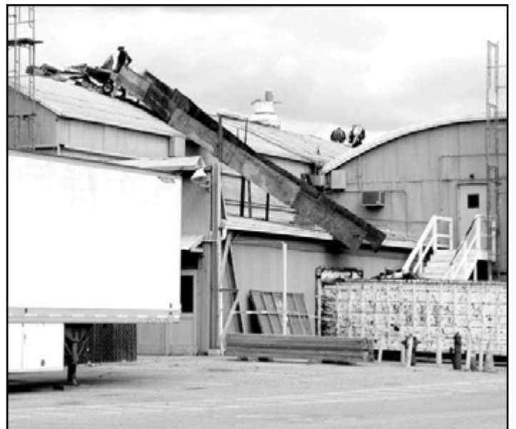
Roofing contractor removes roof materials at Downey Studios while film crews work inside unprotected.
